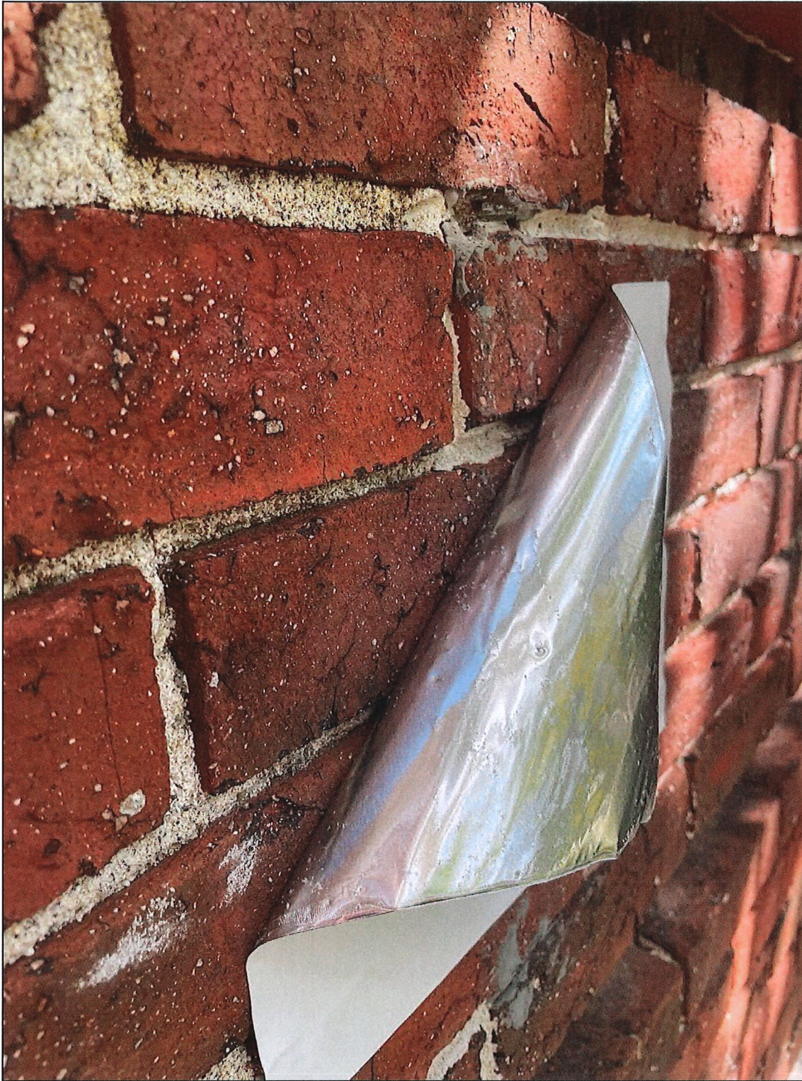
Image 6: Knafel Center south façade test site with sample sign. When removed, thin layer of adhesive very seldom remains (no adhesive is stuck to the wall in this image), but the manufacturer recommends using non-abrasive soap to dissolve any remaining adhesive should that occur.
