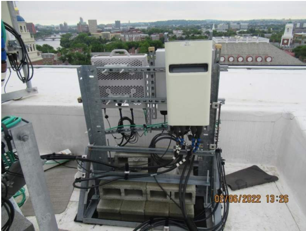
Photo 5: Sample photo illustrating an existing block-style RRH ballast sled.
