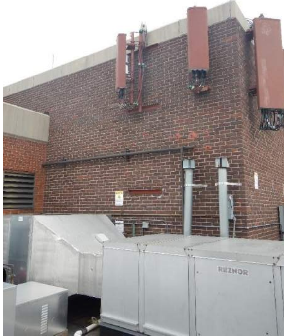
Photo 1: Sample photo illustrating the existing Alpha sector antennas.
