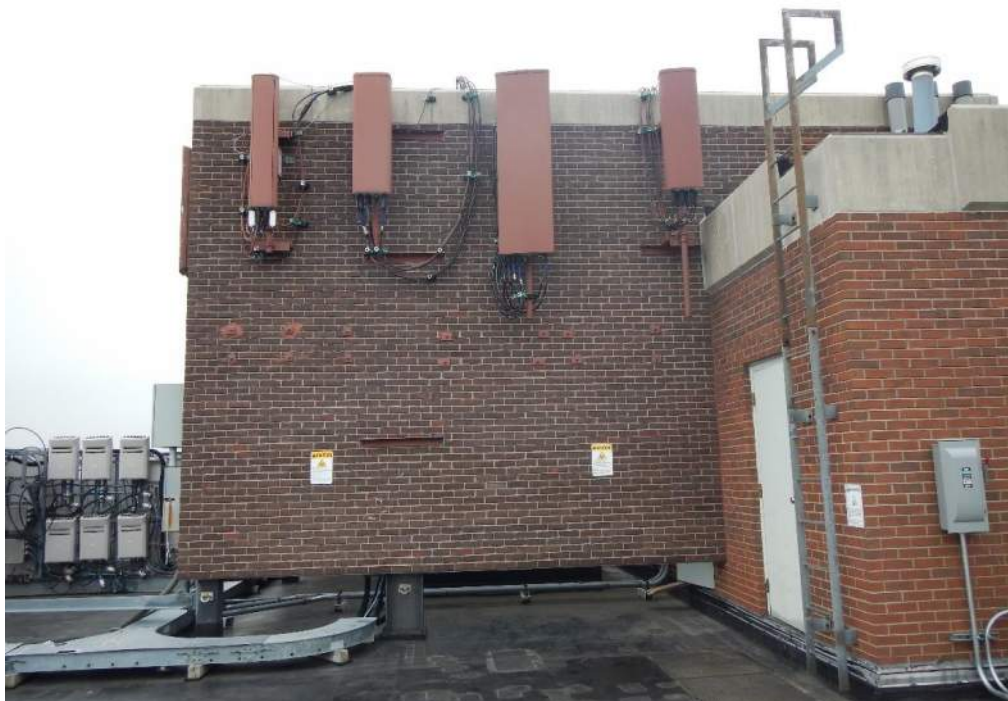
Photo 2: Sample photo illustrating the existing Beta sector antennas.
