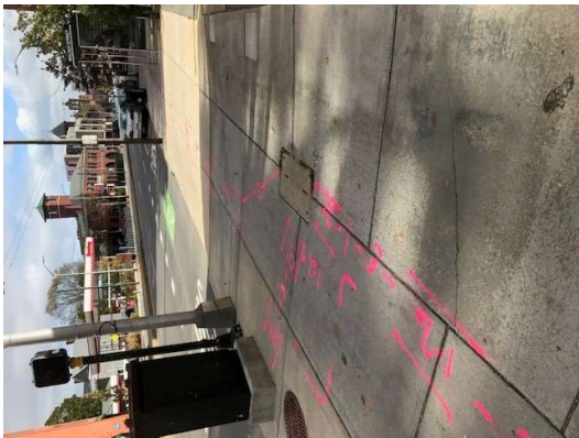
Possible signal control or site lighting located 1-2 feet from the surface, extending in both directions down Mass Ave.
