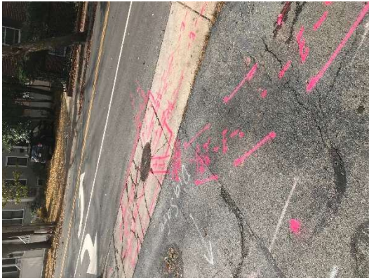
Secondary electrical line to the building exits at 1.5-2 feet and enters the building under the concrete ramp area.
