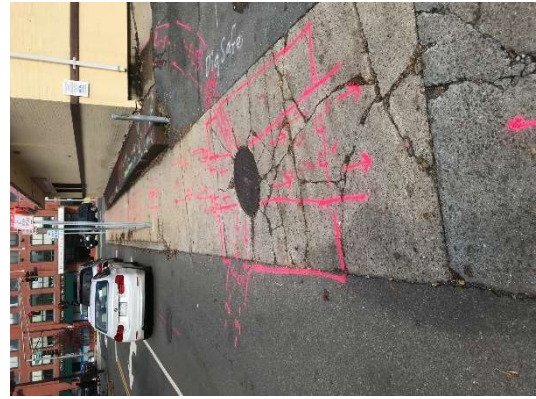
Primary electrical line exits this manhole at 2.5-3 feet from the surface and travels up the sidewalk at a depth of 3.5-4.5 feet.
