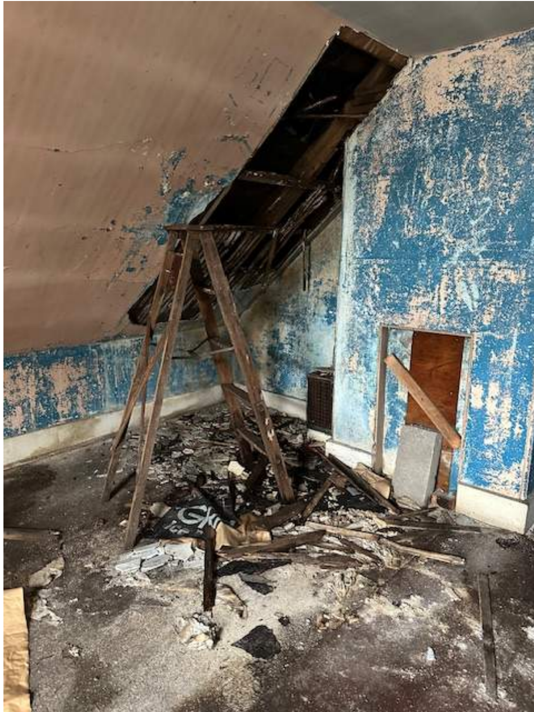
SUBSTANDARD ROOF FRAMING
