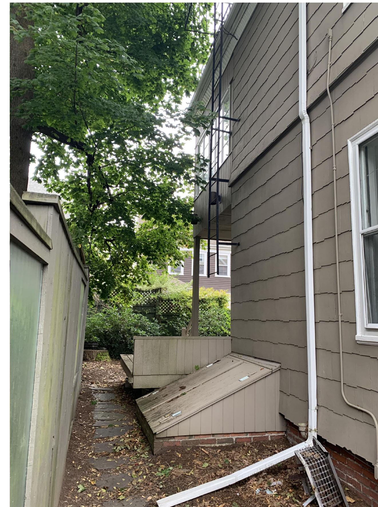
VIEW OF PORCH FROM BACKYARD LOOKING WEST AND OF EXISTING WINDOW TO BE SHORTENED AND SLIGHTLY ELEVATED
