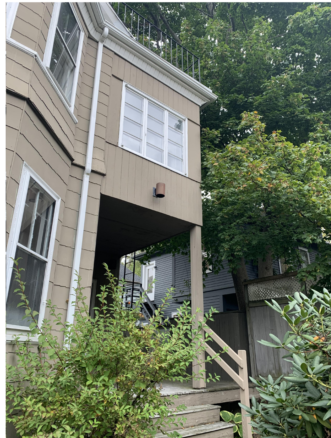
VIEW OF PORCH LOOKING AT WEST ELEVATION @ BACK OF HOUSE: EXISTING COVERED PORCH
