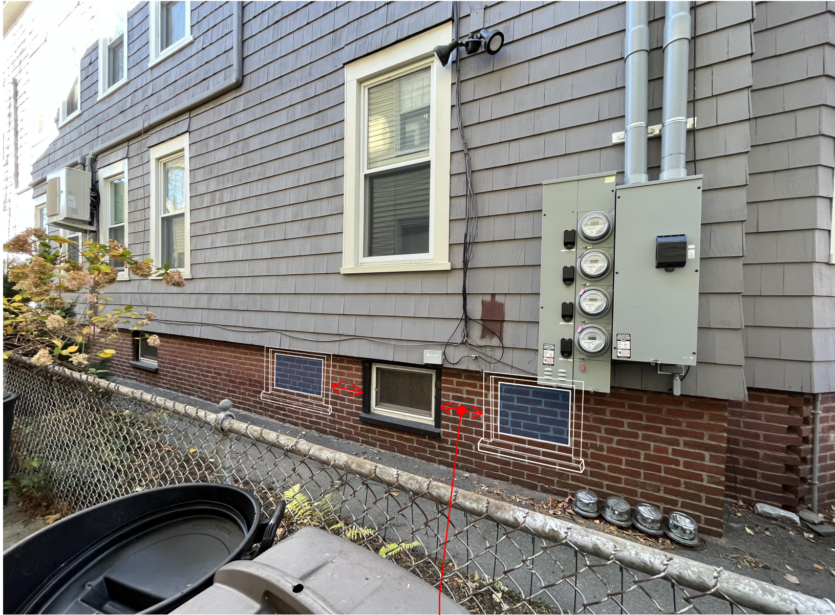
2 new windows, masonry opening spaced 2 bricks (16") from existing window. Windows match size and height of existing windows. Trim to match existing.
