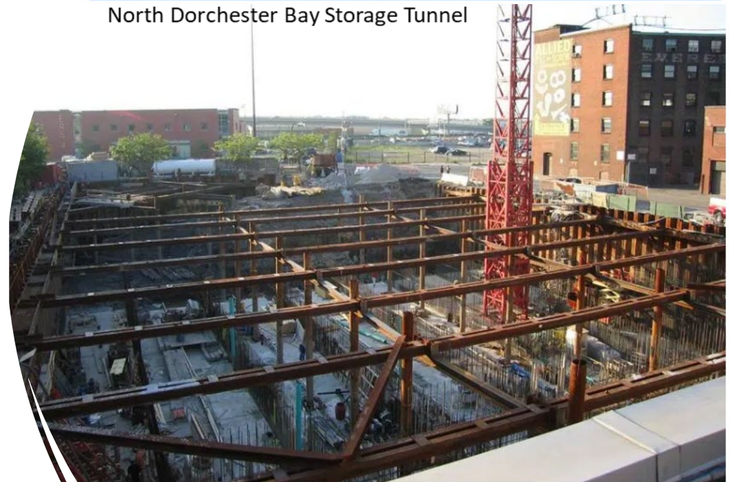
Union Park CSO Facility Storage Basins: Photo Credit: Simpson Gumpertz & Heger (SGH) https://www.sgh.com/project/union-park-detention-facility/
