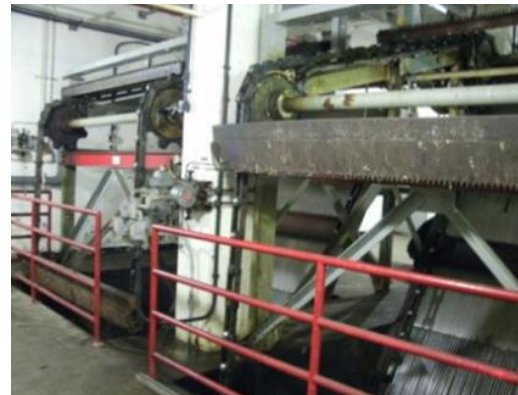
Mechanical Bar Screens
