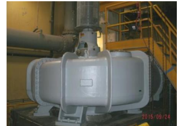
Wet Weather Pump
