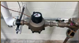
Typical Water Meter.
