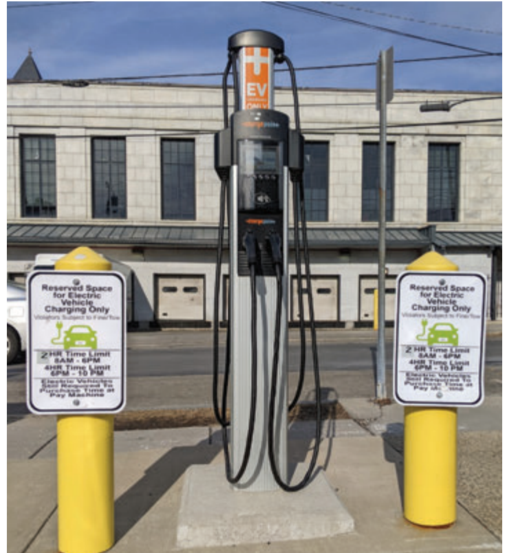
Electric Vehicle charging station on Green Street
