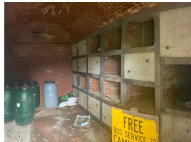
Receiving Tomb interior is deteriorated and underused.
