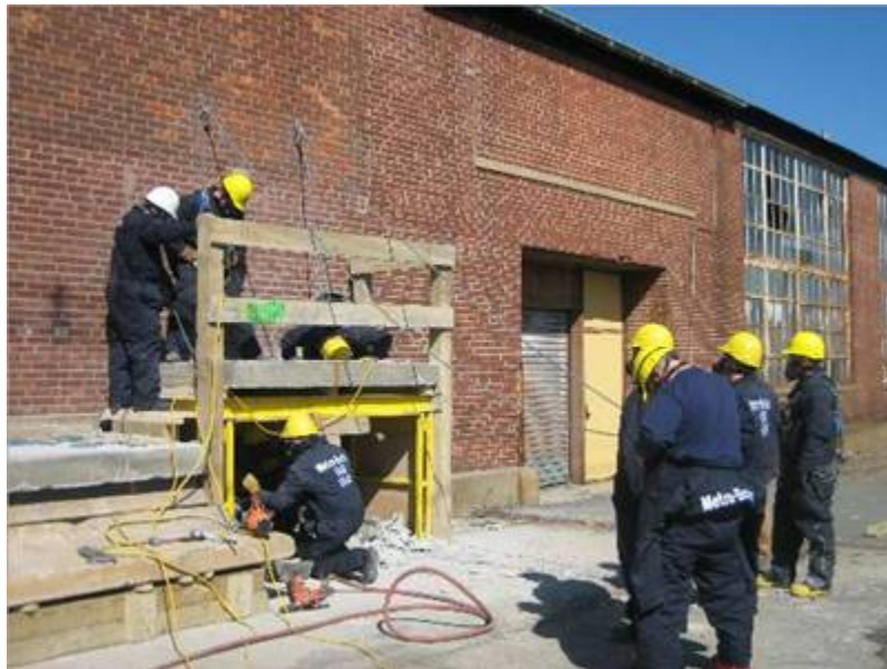
Pneumatic tool station
