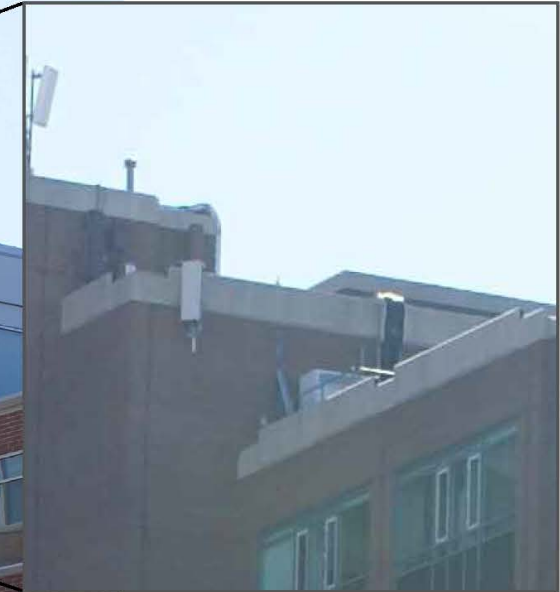
DETAIL OF EQUIPMENT
