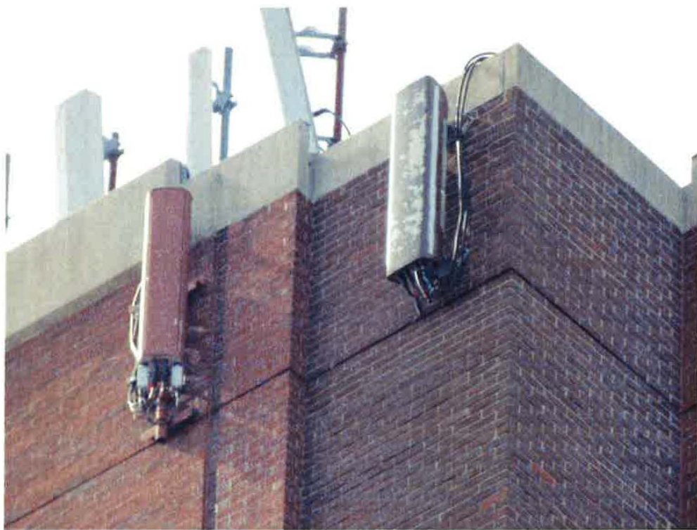
Photo 1: Sample photo illustrating the existing alpha sector antennas.
