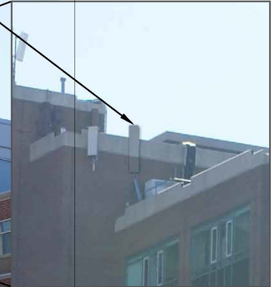
DETAIL OF EQUIPMENT
