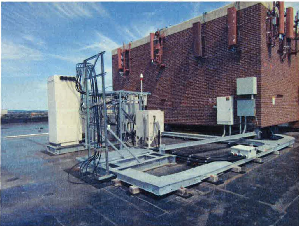
Photo 4: Sample photo illustrating the existing equipment.
