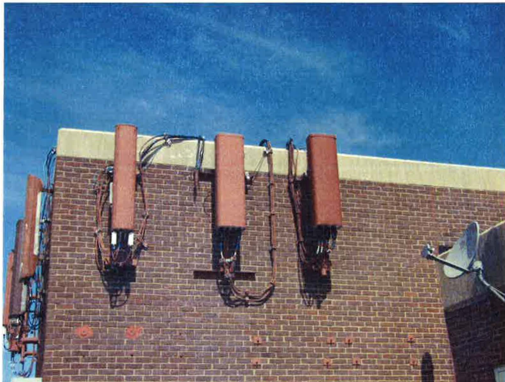
Photo 2: Sample photo illustrating the existing beta/gamma sector antennas.
