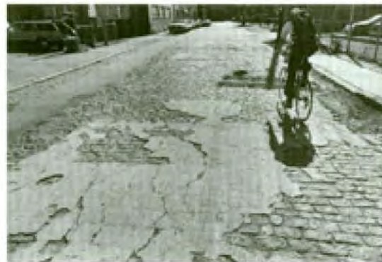
Many of the streets and sidewalks are in disrepair.
