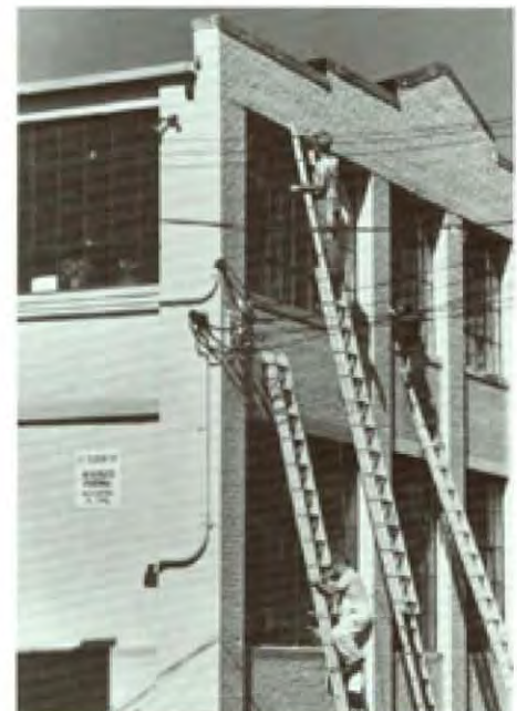
Upholstery Modes, a furniture manufacturing company, renovated its turn of the century industrial building in 1982.
