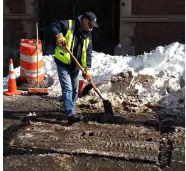
DPW staff secure a roadway steel plate by placing asphalt around the edges
