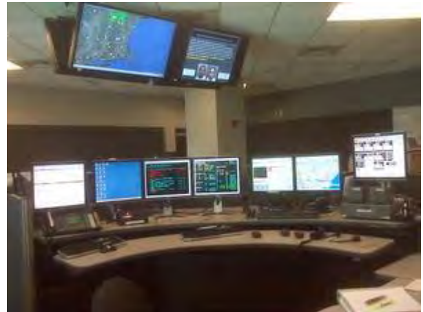
Public safety communications equipment
