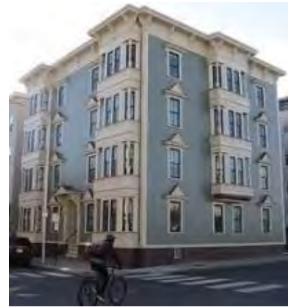
The first of four buildings to be rehabbed as part of the preservation of Bishop Allen Apartments, a 32-unit affordable development
