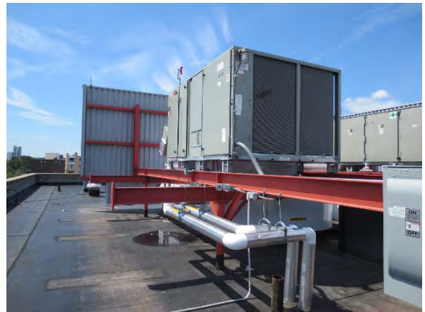
Public Works upgraded HVAC equipment on the Citywide Senior Center roof this year.
