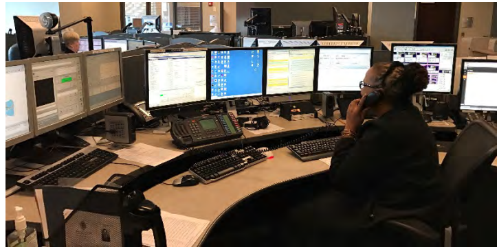
Inside the Emergency Communications Center (ECC).
