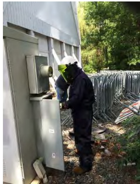
Electrical staff testing equipment.
