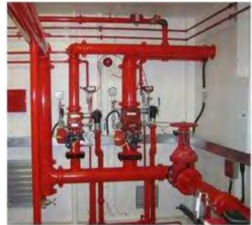
The duties of the Cambridge Fire Prevention Bureau include inspecting fire detection and alarm systems.
