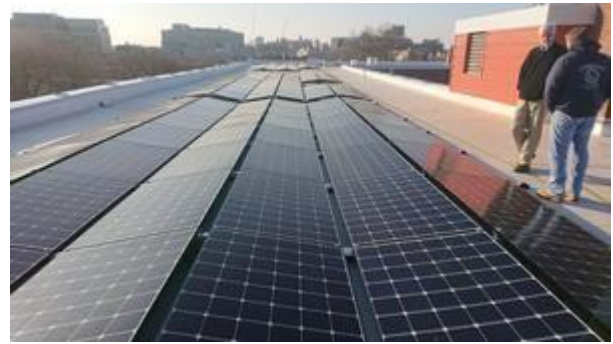
A new 97kW AC Solar Photovoltaic array installed at the Fletcher Maynard Academy
