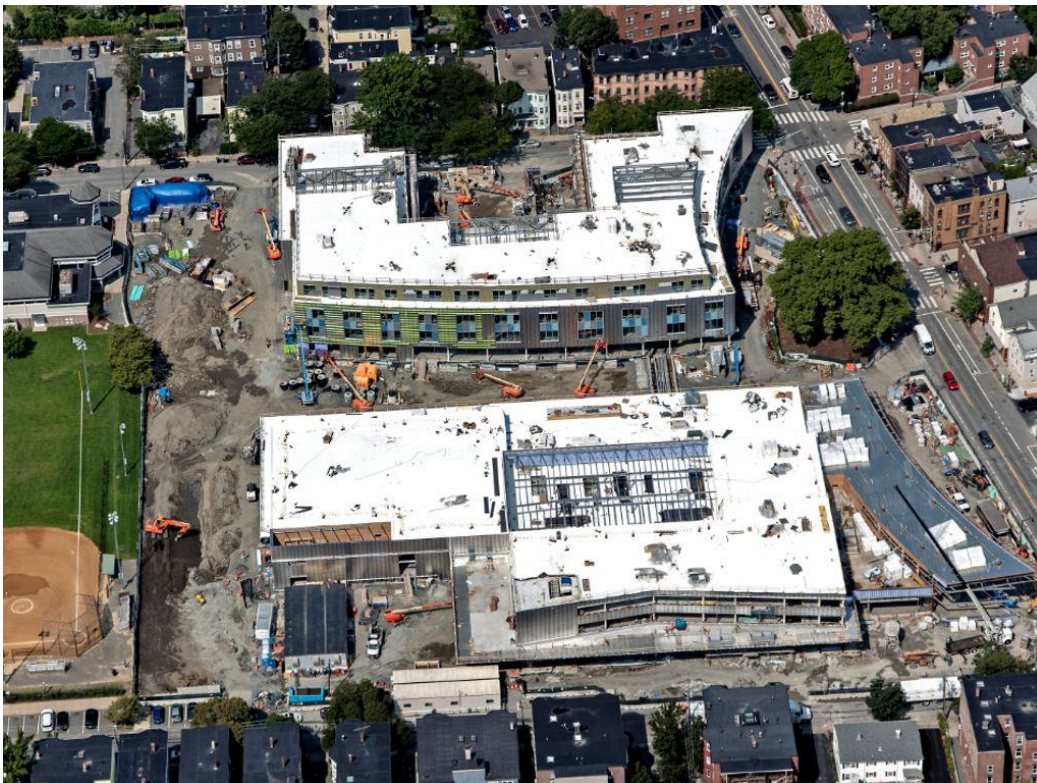
Construction of the King Open and Cambridge Street Upper Schools and Community Complex, August 2018
