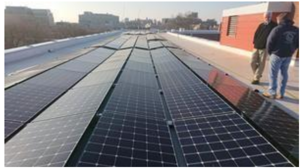
A new 97kW AC Solar Photovoltaic array installed at the Fletcher Maynard Academy
