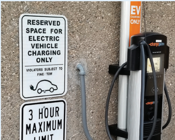
Electric Vehicle Charging Station
