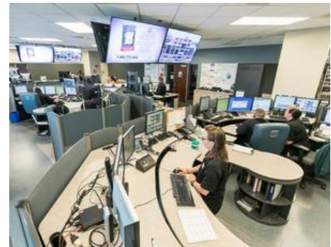
Emergency Communications Center
