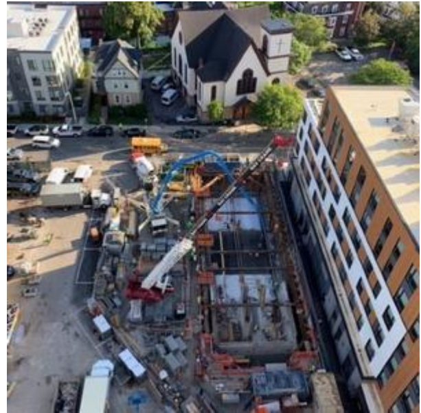
Construction of a stormwater tank on Bishop Allen Drive associated with The Port Infrastructure Project
