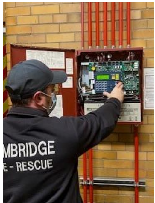
A member of Fire Prevention inspecting/testing a Fire Alarm Control Panel
