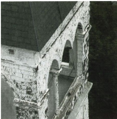
Deteriorated belfry finishes; missing column; damaged siding and trim.
