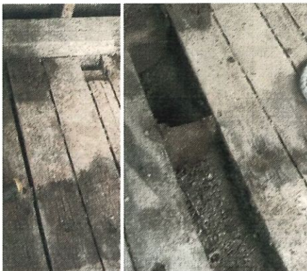
Hazard Under Floor Boards
