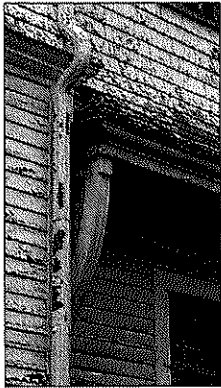
DAMAGED DOWNSPOUT AND SHINGLE HOOD AT WEST FRONT
