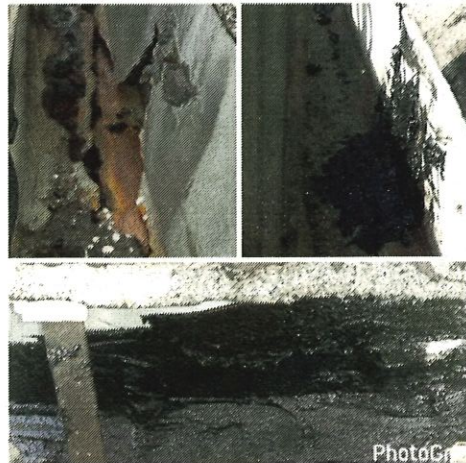
Temporary Repair - Gutter
