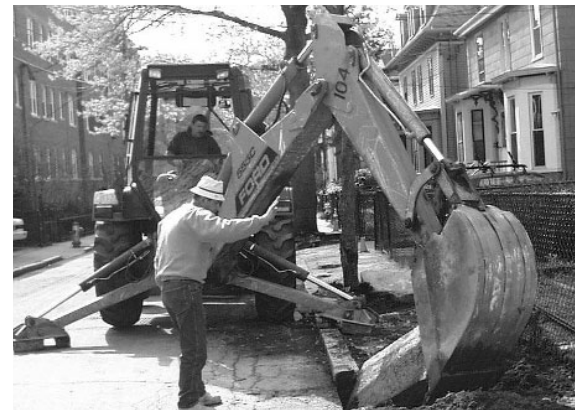
Construction Division employees removing curbing from a sidewalk in Cambridgeport in preparation for the installation of a curb-cut.
