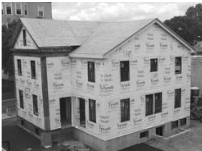
Just A Start began construction at Scouting Way, where new construction, combined with renovation of an existing historic structure, will create 13 affordable family-sized rental units adjacent to Sennott Park.
