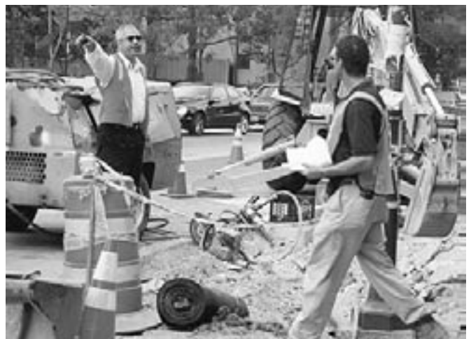
Public Works employees provide construction management and oversight for the Cambridge Street Improvement Project.
