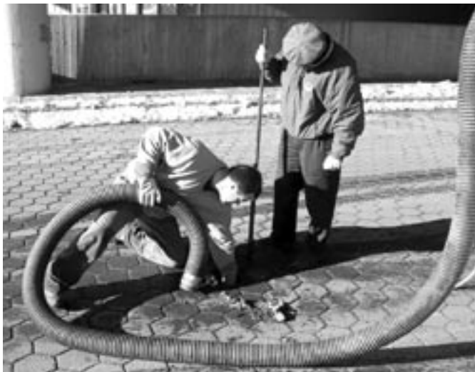
Hector Perez and Ed Sennott put the finishing touches on a water service repair necessary to keep the water transmission and distribution system working safely.
