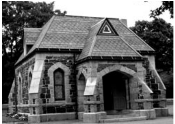
Exterior façade repointing at the Cemetery chapel was completed with the assistance of funding from the Community Preservation Act.
