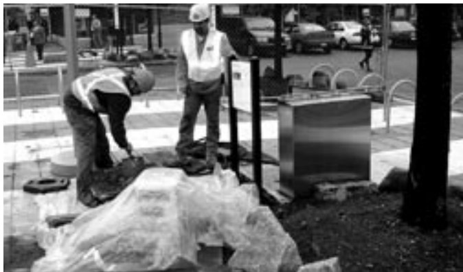
Workers install a marker at Porter Square commemorating the history of the Rand family estate, which occupied the site for a century before it became a shopping center.
