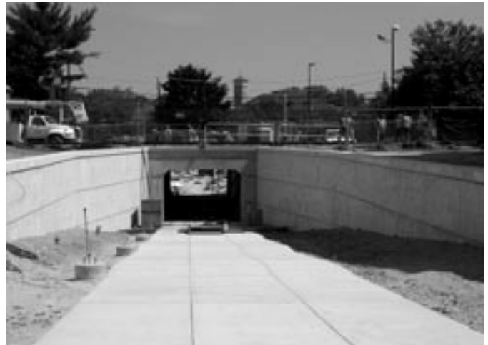
Construction is nearly completed on the Yerxa Road Pedestrian Underpass, which will provide a safe, accessible connection between Walden Square and the Peabody School, as well as landscape and drainage improvements. [Credit: Katherine Watkins]
