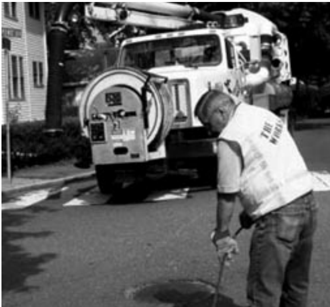
Routine sewer and drain maintenance is part of the DPW's continuing effort to institute best management practices for stormwater management.
