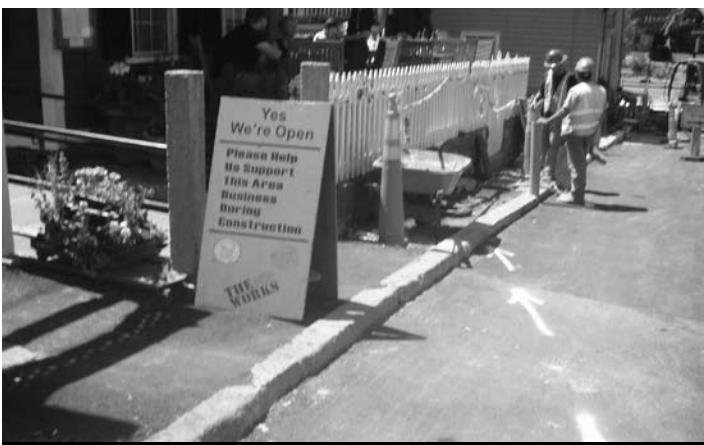
Construction on Winthrop Street, part of the Harvard Square Improvement Project. [Photo Credit: William Dwyer]
