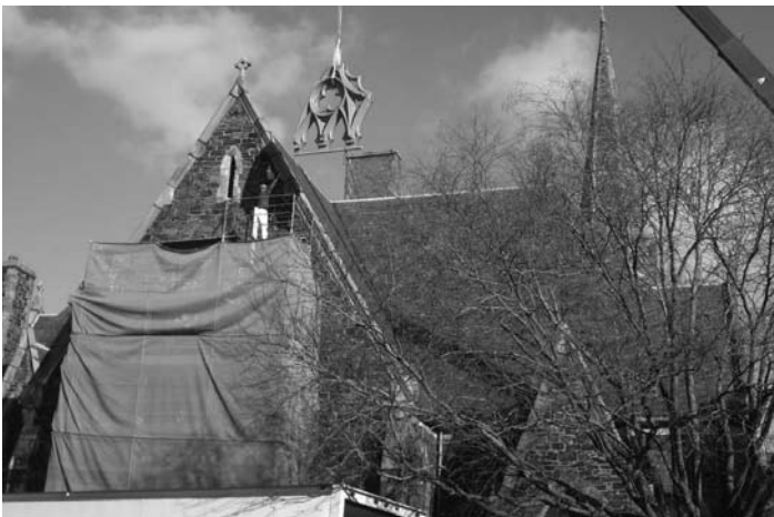
Contractors reinstall a restored Tiffany window and frame at the Old Cambridge Baptist Church, with financial support from a Community Preservation Act-funded Institutional Preservation Grant.
