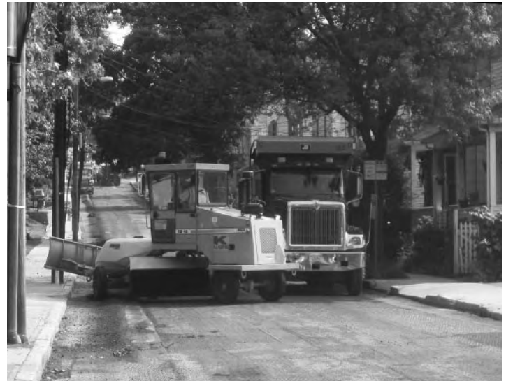
DPW maintains and repairs over 125 miles of streets. Last year, the department completed 450 pothole repairs, 159 other street repairs, and resurfaced 5 streets.
