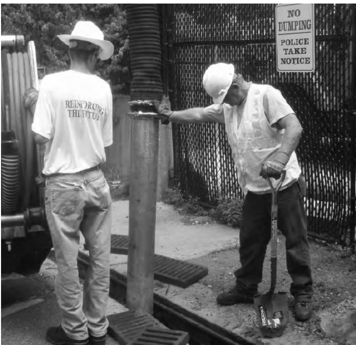
Last year, the Street and Sewer Division cleaned 2,200 catch basins as part of the DPW's continuing effort to institute the best management practices for stormwater management.
