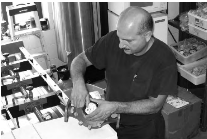
Phil Sciandra prepares a water meter for installation. Photo by Ralph Dunphy
