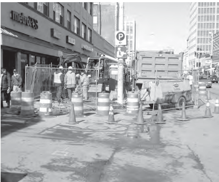
DPW managed construction of major public infrastructure projects, including the Central Square Manhole Separation Project.
