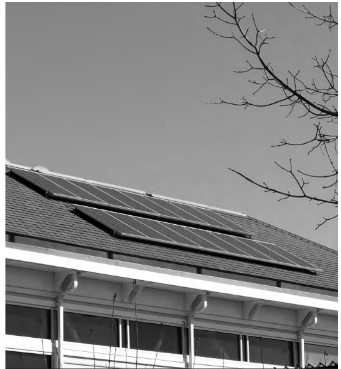
Several City buildings received photovoltaic panel systems this year. The Frisoli Youth Center panel system pictured here, will generate 3.26 kilowatts that will feed back into the grid.
