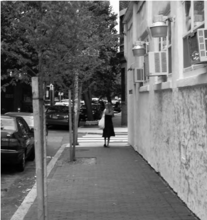
This year, the Engineering Division replaced 8.5 miles of sidewalk, including this one on Harvard Street at Pine Street.
