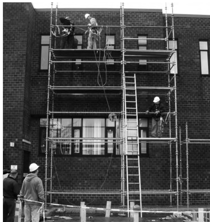
The Public Buildings Division includes Construction, Maintenance, and Operations Divisions. Here, crews perform façade repairs on the Frazier Building at DPW.
