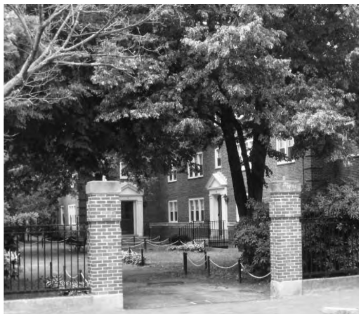
Comprehensive renovation of 45 housing units is under way at Jackson Gardens in Mid-Cambridge.
