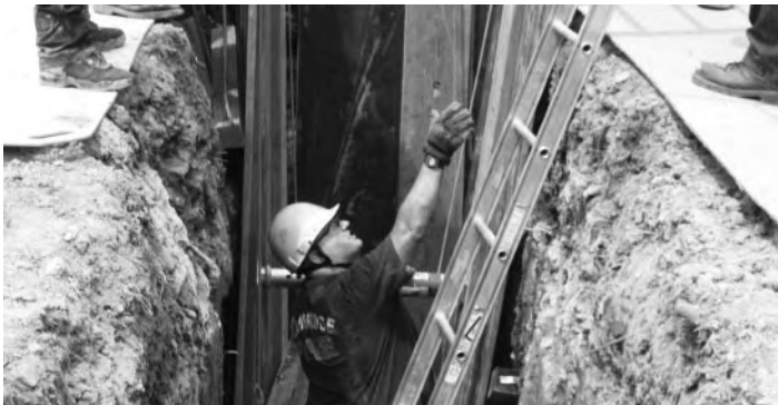
Members of the CFD Technical Rescue Team review skills and safety procedures in trench shoring and collapse rescue. (Photo by Tara Bithia)
