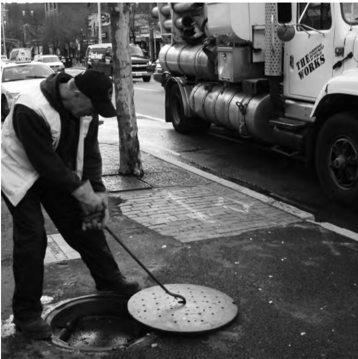
The Sewer Maintenance Division maintains over 223 miles of sewer and stormwater lines, more than 6,000 catch basins and 33 sewer and stormwater pump stations.
