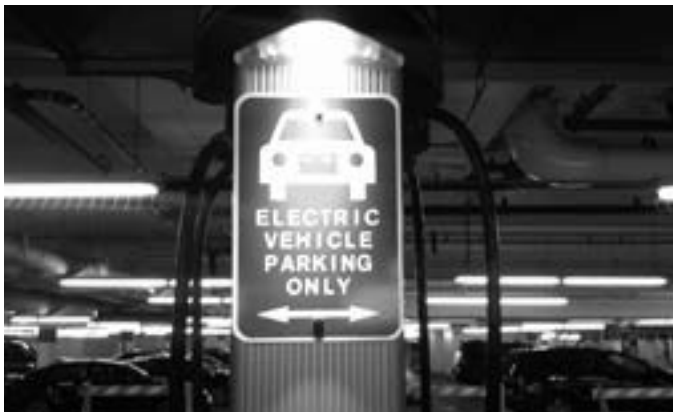
To encourage the use of electric vehicles, Cambridge joined a national network to install charging stations at publicly accessible locations citywide, including the Cambridge Center West Garage in Kendall Square.
