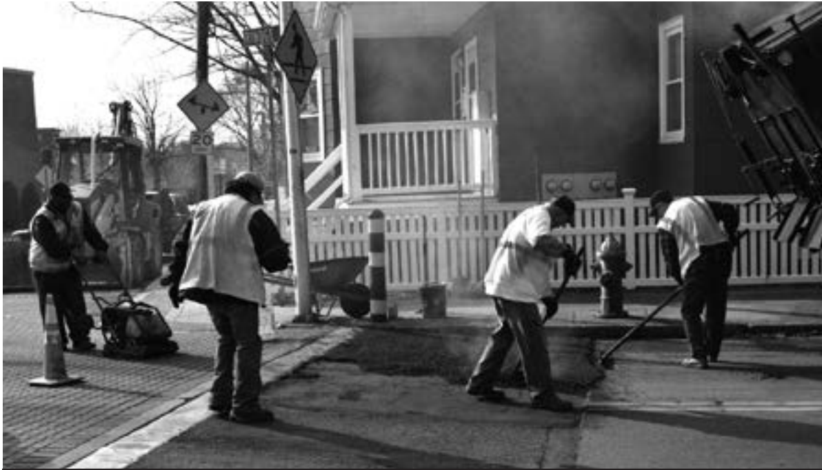
Streets and Sidewalks Maintenance crews perform inspections and repairs throughout the city. Here, crews perform repairs on the raised intersection at Rindge Avenue and Yerxa Road.
