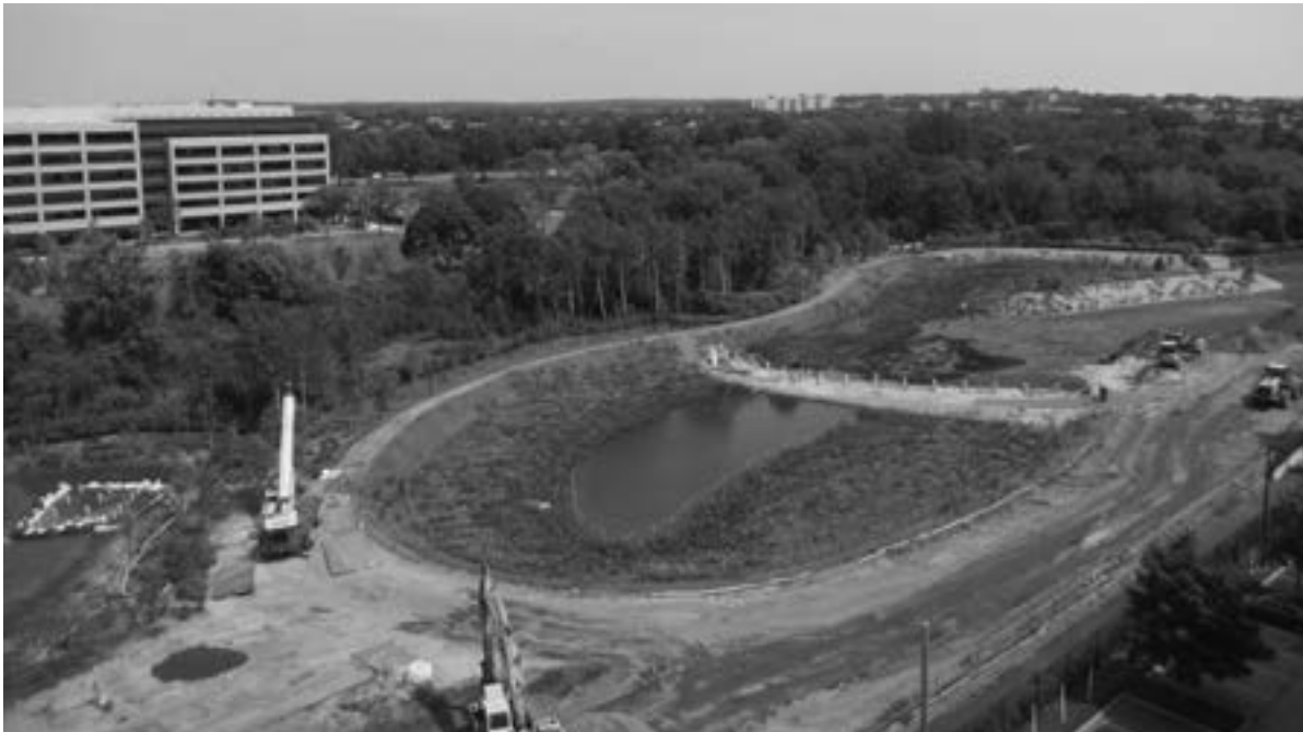
The Engineering Division oversees construction projects in the City, such as Cambridgepark Drive Area Drainage Improvements and Stormwater Wetland Project (pictured). When complete, the project will provide significant environmental benefits by minimizing flooding and protecting Fresh Pond and Alewife Brook.
