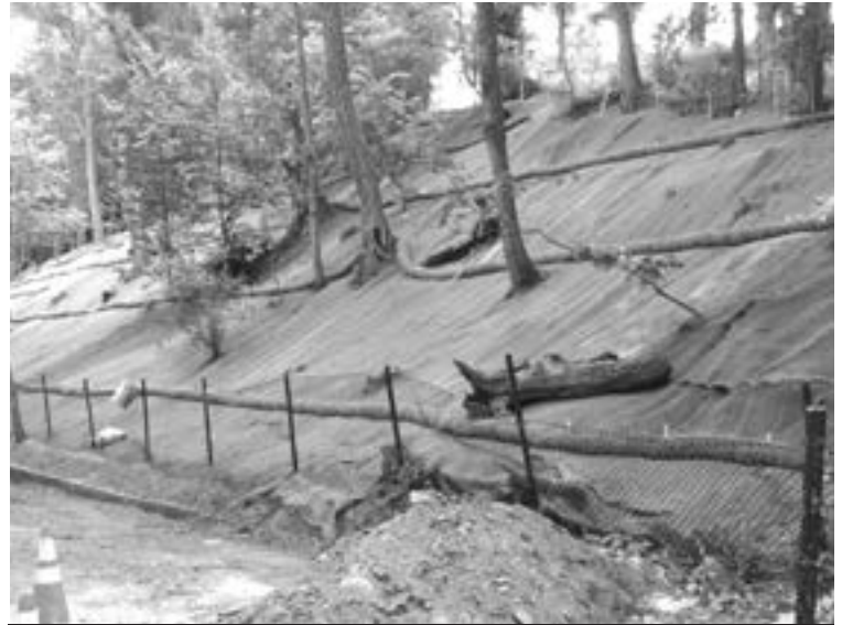
Work is in progress on Phase III of the Glacken Slope Restoration Project.
