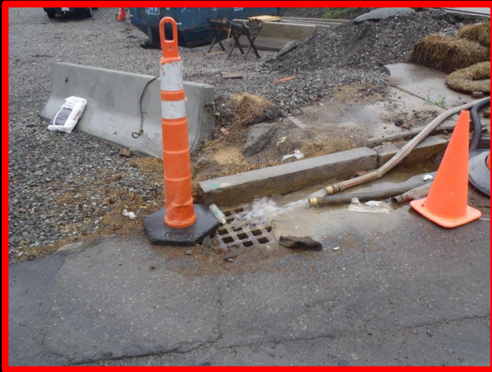
Hose to Catch Basin
